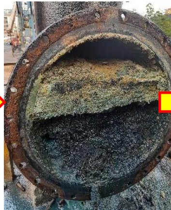
COG Pipe choked with Solid Muck
