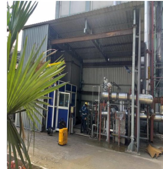
Site Pic of Micro Turbine, CDQ, TSK
